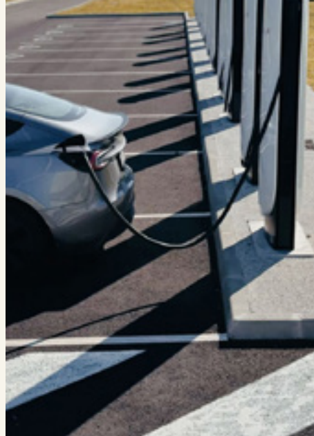
Electric Vehicle Chargers/ Future-ready convenience
